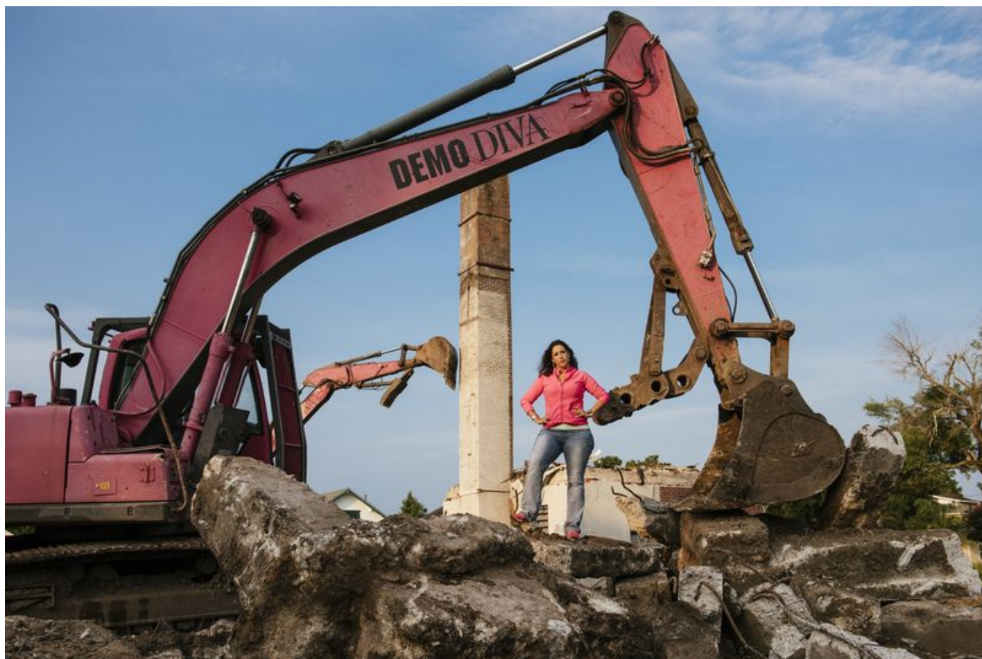
Simone Bruni, on a job site in New Orleans. Her excavator is named "Smashing Star," because "she looks smashing." (Rush Jagoe)
